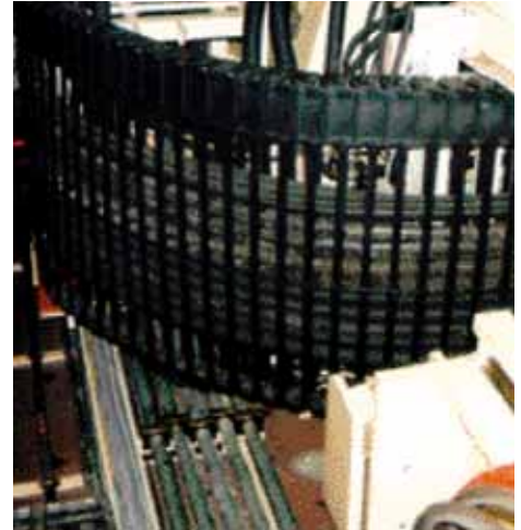
Hydraulic and electrical systems (in closed section) are separated from one other in this example.
