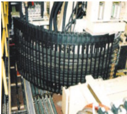
Hydraulics and electric cables are separated from one another in this example
