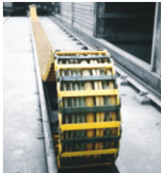
E4 in a pre-cast concrete plant with dust and concrete sediment
