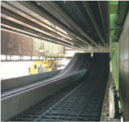
Assembled system in a ship unloading crane with igus® 5050RHD - Travel 106 m, Speed 4 m/s, Fill weight 25 kg/m
