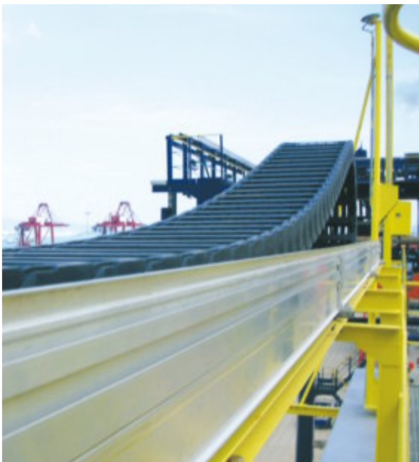
Seawater resistant super-alu-trough in a RTG-crane. Long travel with the E4/4 system
